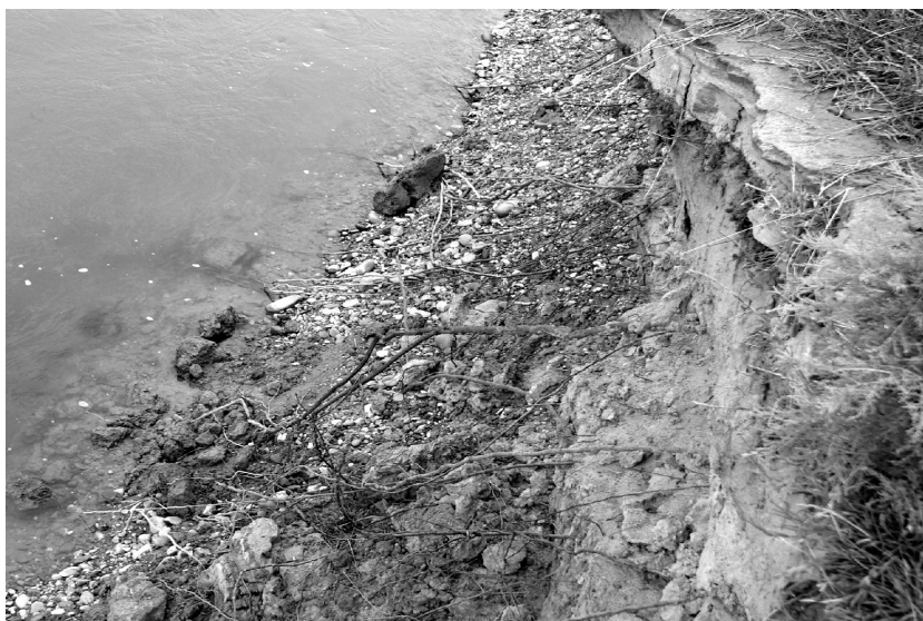
Fig. 4. The stabilization of the banks of the Trotus mouth at Siret river is inefficient. Buckthorn is recommended.
