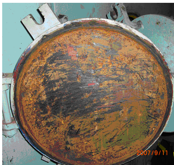
Fig 2. Fouling on the down front cover of the steam condenser
