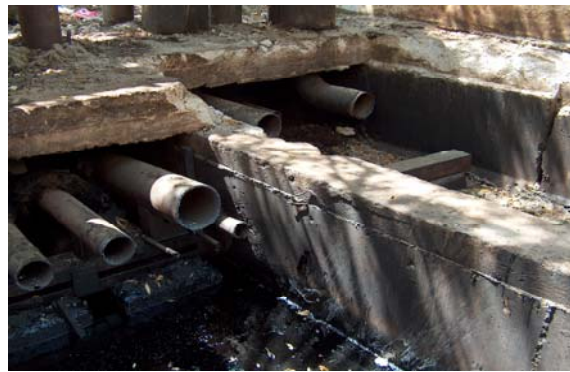
Fig. 1 – Generals aspect of the location – access to the failure zone
