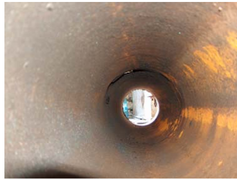
Fig. 3 - The failure zone – internal detail
