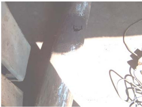
Fig. 2 – The failure zone – external detail
