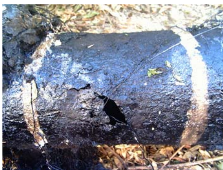
Fig. 7 – The external detail, failure
