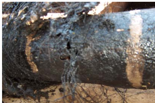
Fig. 4 – The failure zone – external detail, traces of protective system
