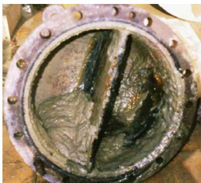
Fig. 2. Sediments accumulation in water boxes
