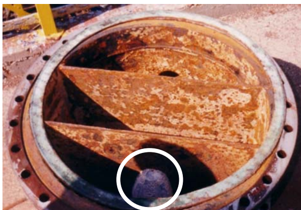
Fig. 8. Water box of a heat exchanger protected with zinc sacrificial anode
