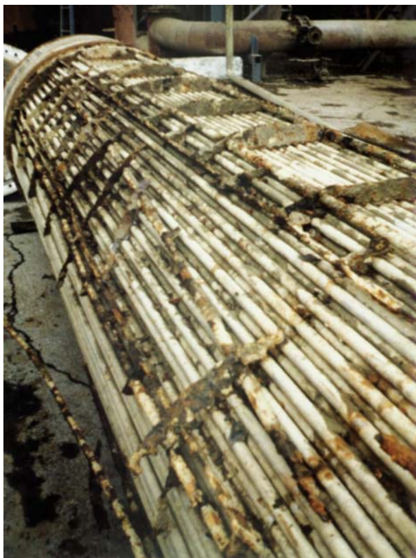
Fig. 7. Mild steel baffles and rods severely corroded in chemically treated water due to the contact with stainless steel tubes bundle
